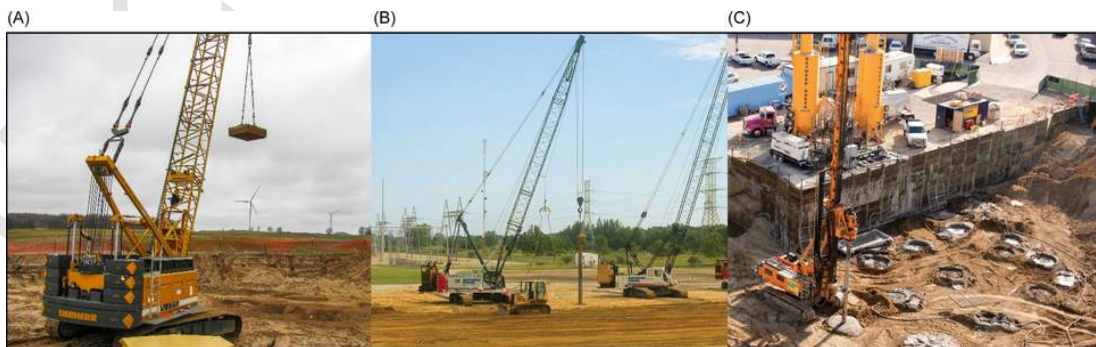
Fig. 12 Examples of soil improvement technologies: (A) deep dynamic compaction, (B) vibro compaction, and (C) deep soil mixing. Photographs courtesy of Keller.
